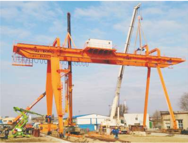
Lifting gantry crane of load capacity 50t in the design position. Spetsmost, Moscow
