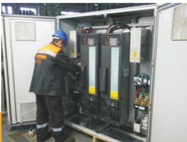
Assembly of electrical cabinets based on "Siemens"
