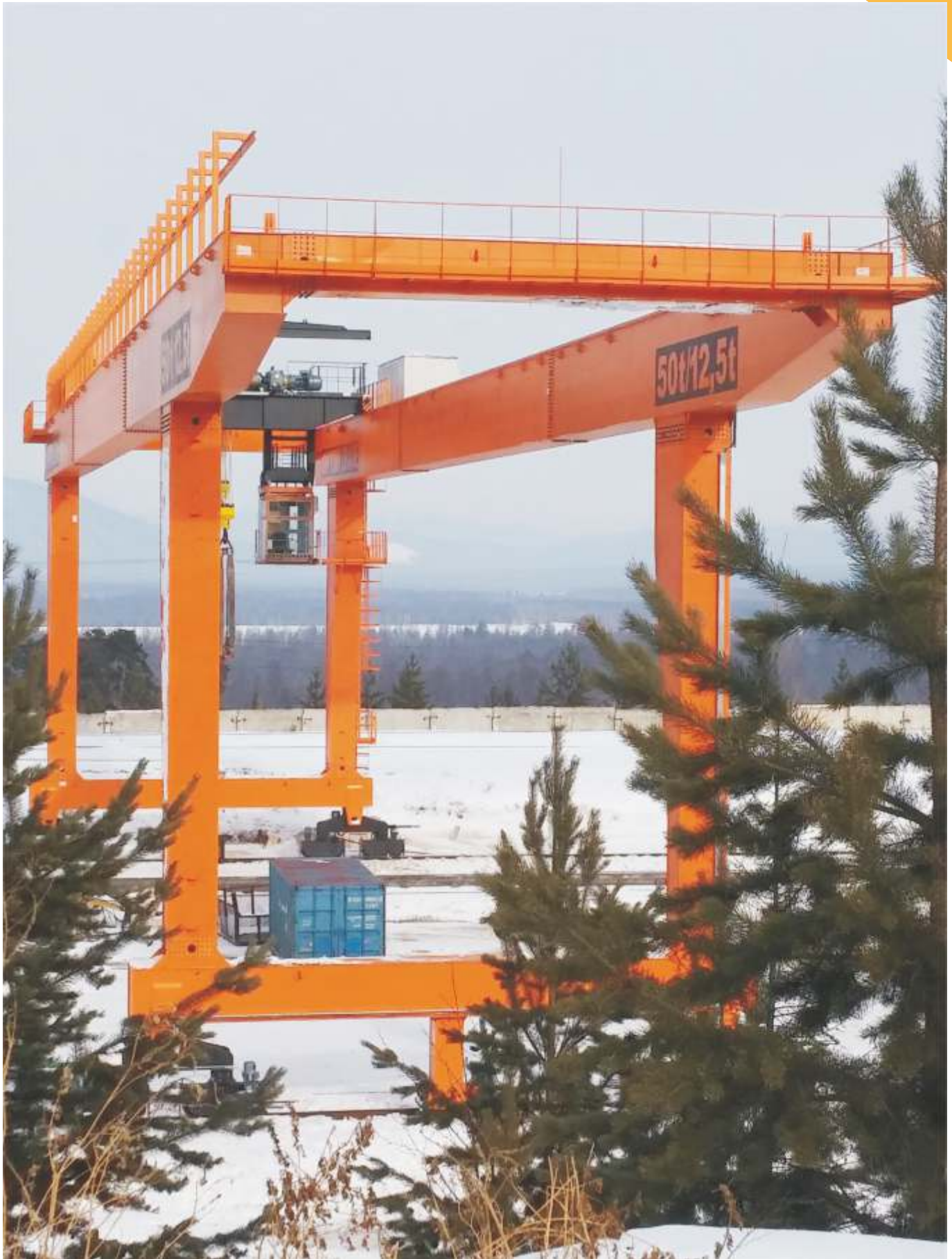
Gantry crane of load capacity 50/12,5 t, span – 46 m. Polyusgold, Yakutia.
